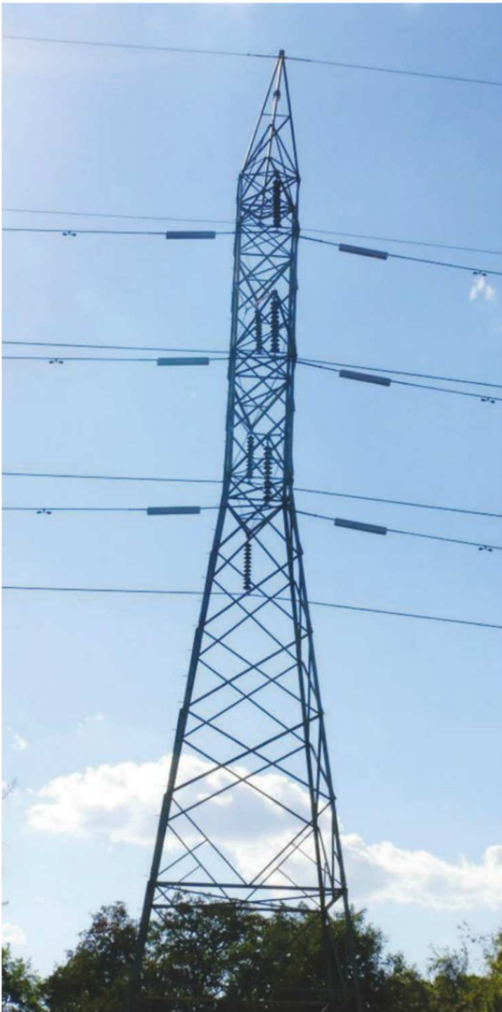
TVA installed 99 DSRs on this 161-kV transmission line to demonstrate the control capability provided by these units.
